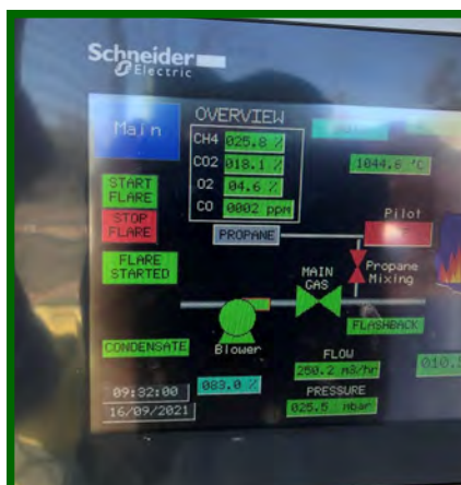
Control panel of flare operating
