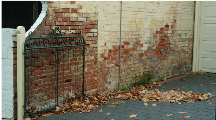
Rising damp on a painted brick wall in Norwood.
