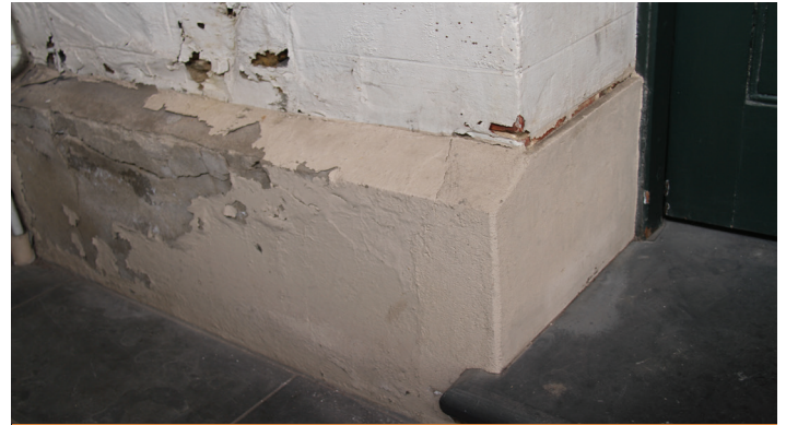
Rising damp exacerbated by hard cement render repairs.
